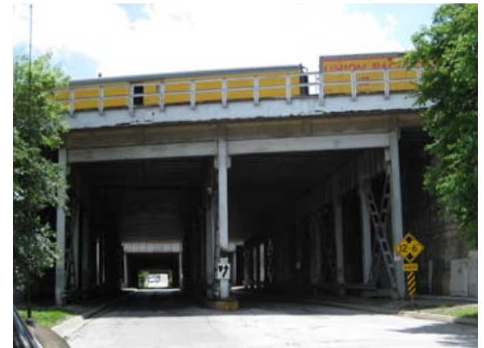
7th Street underpass connecting the South Riverfront with the Near South District
